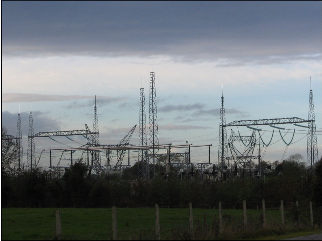
Figure 3.3 Oldstreet 400kV Station
